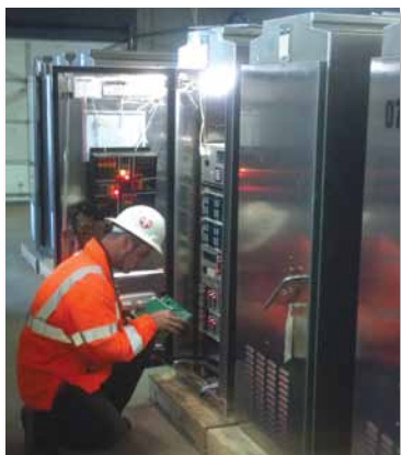
Signal Mechanic Greg Carter of ALS of North Carolina verifies conflict monitor settings during controller cabinet testing just before installing them for the City of Greensboro.
